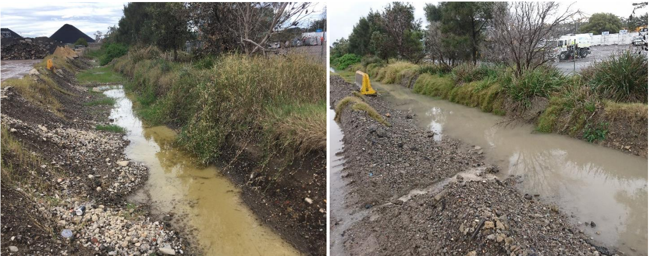
Photograph 2.1 Infiltration swale - the image on the left was taken in March 2019, after 50 to 60 mm of rainfall. Only minor amounts of surface water runoff occurred from this event. The image on the right was taken in August 2019 after approximately 80 mm of rain. Significant surface runoff from the yard occurred from this event.
