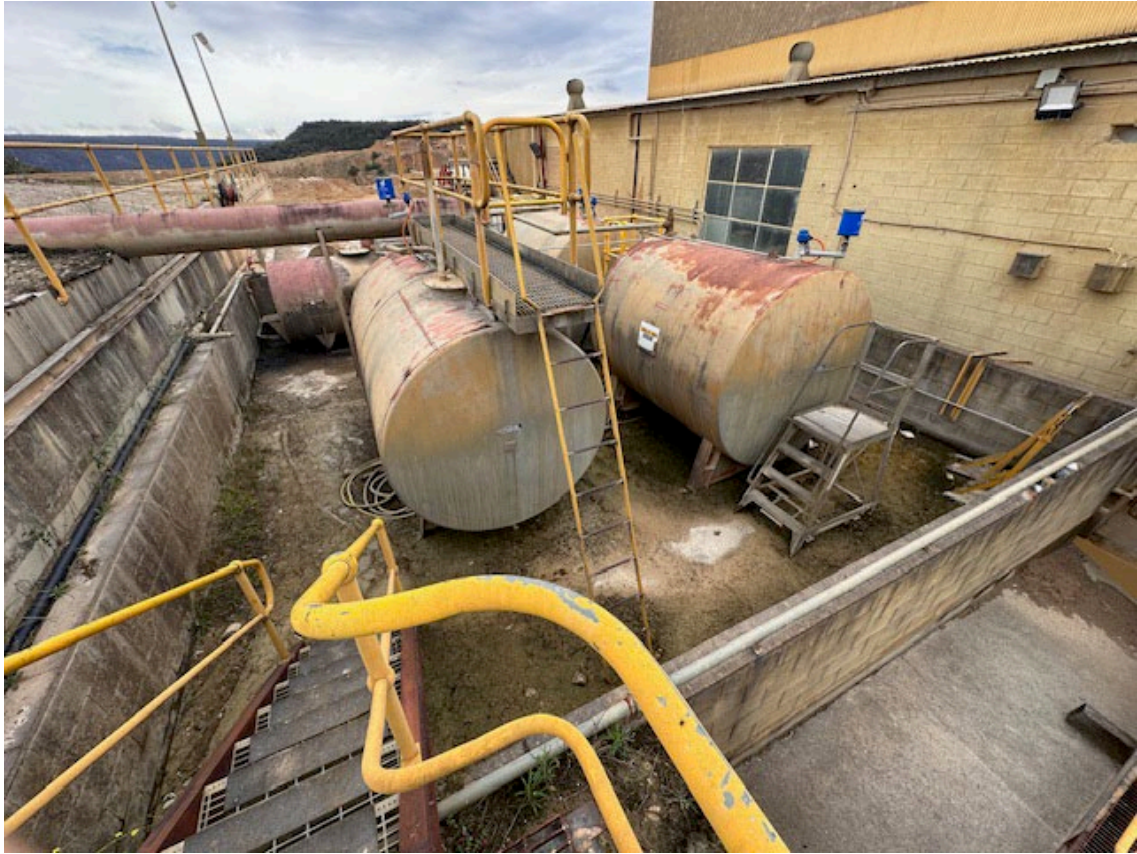
Fuel storage within bunded area at maintenance workshop
