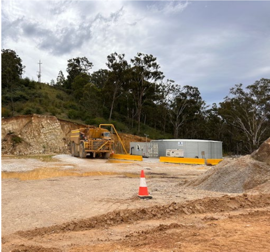
Water cart, with water tank and Polo Citrus dust suppressant dosing station purpose built for dust suppression
