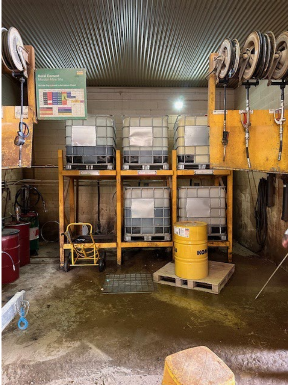
Oil storage in maintenance workshop – within bunded area that connects to oil and water separator
