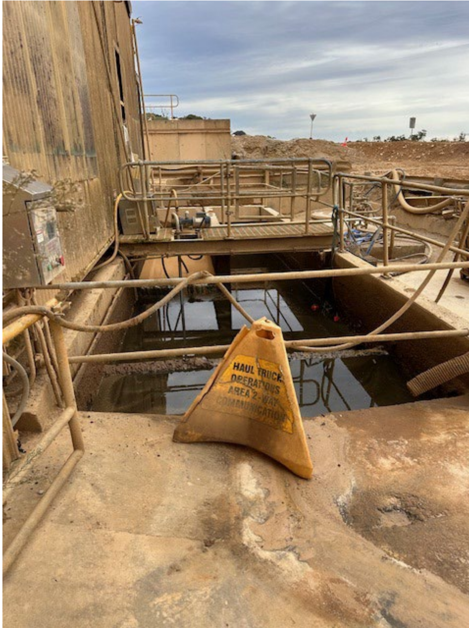
Oil and water separator outside maintenance workshop
