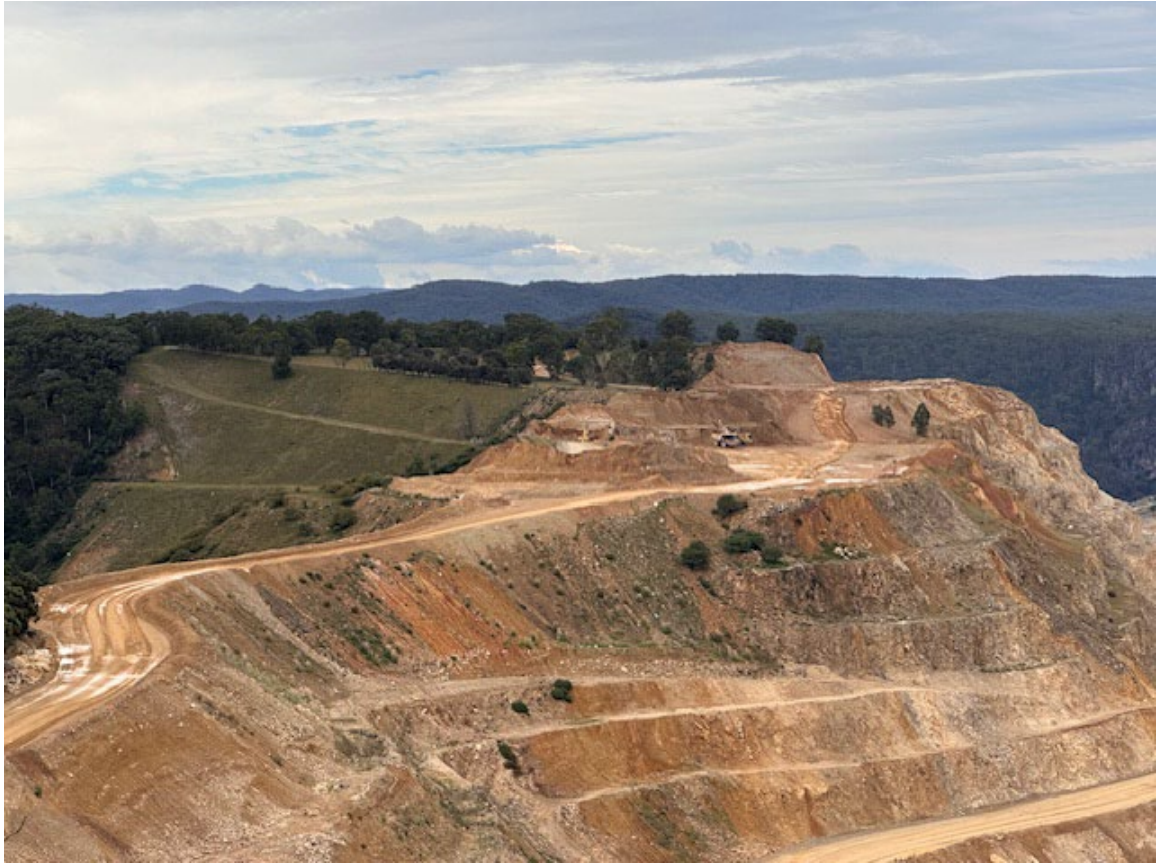
Evidence of slope stabilisation and active amelioration works for Bryce's Gully landslip area on eastern side of mine
