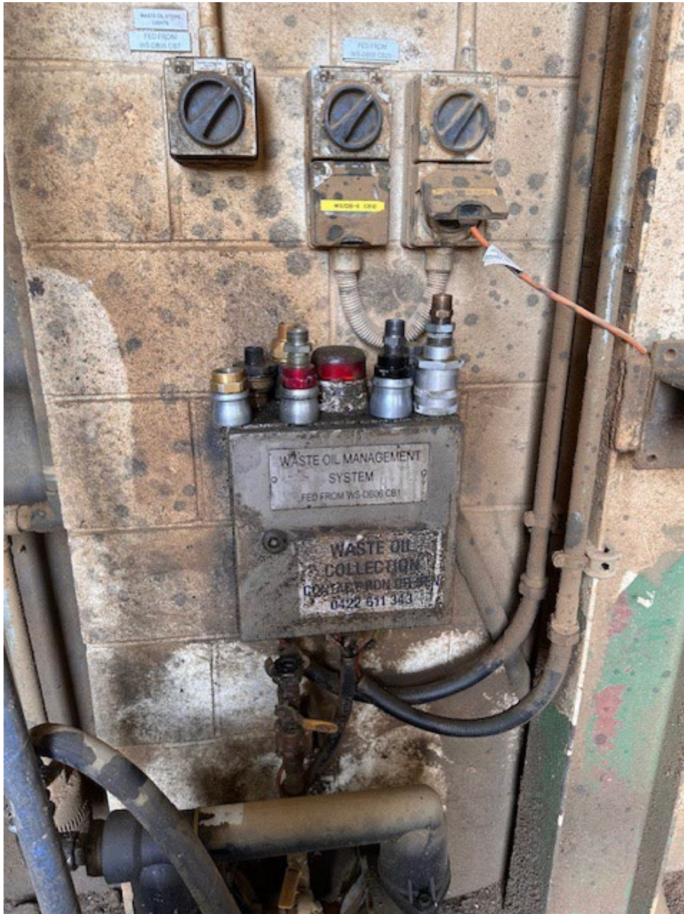
Waste oil management alert system
