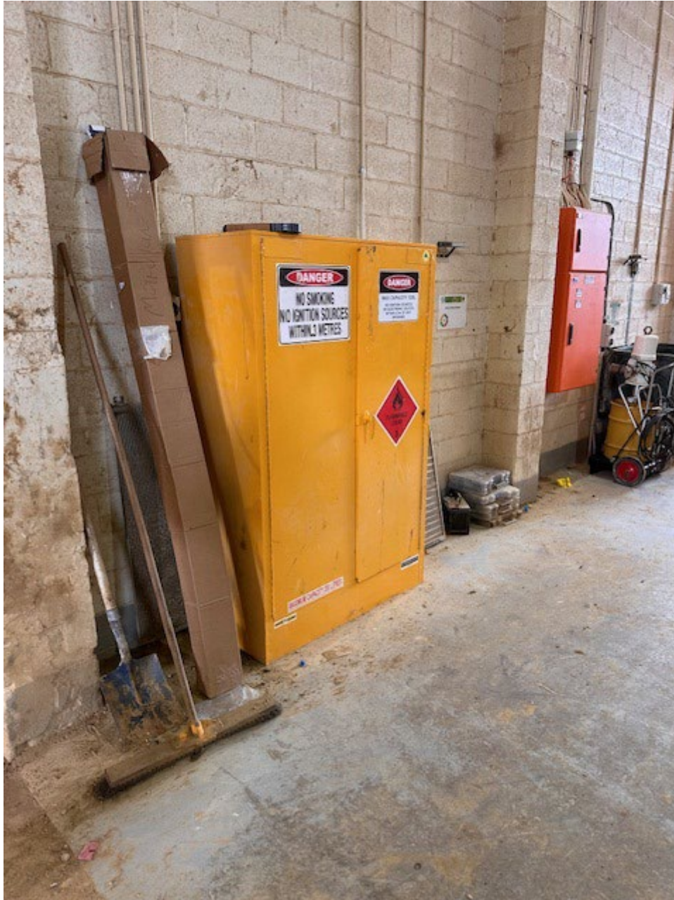
Appropriate storage of flammable goods with signage
