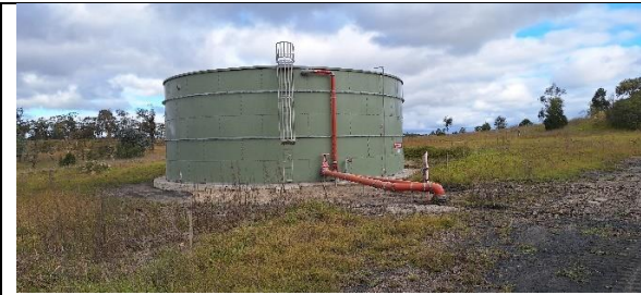
Photo 15 – Firefighting Water Supply Tank
