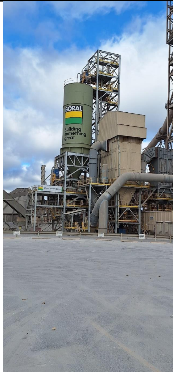
Photo 1 – Bag filters and Chlorine Bypass System
