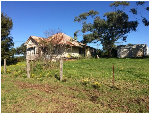
Plate 3. Exposures along fenceline near house on ridge crest. Surface erosion is minor
