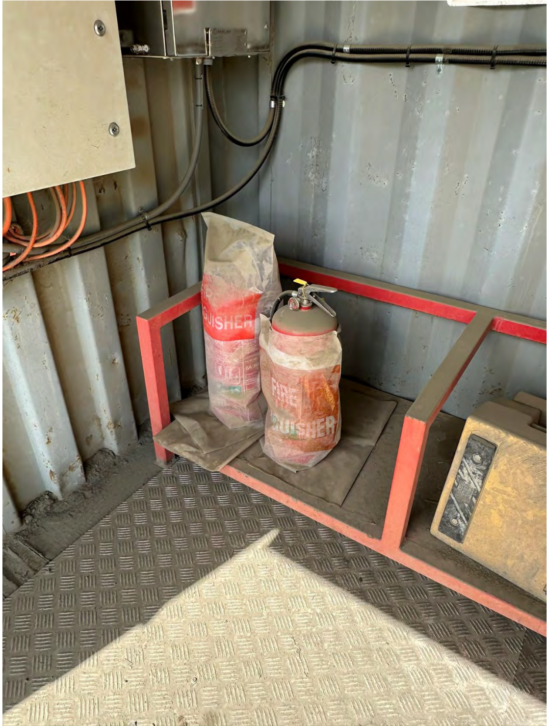
Example of fire response equipment.
