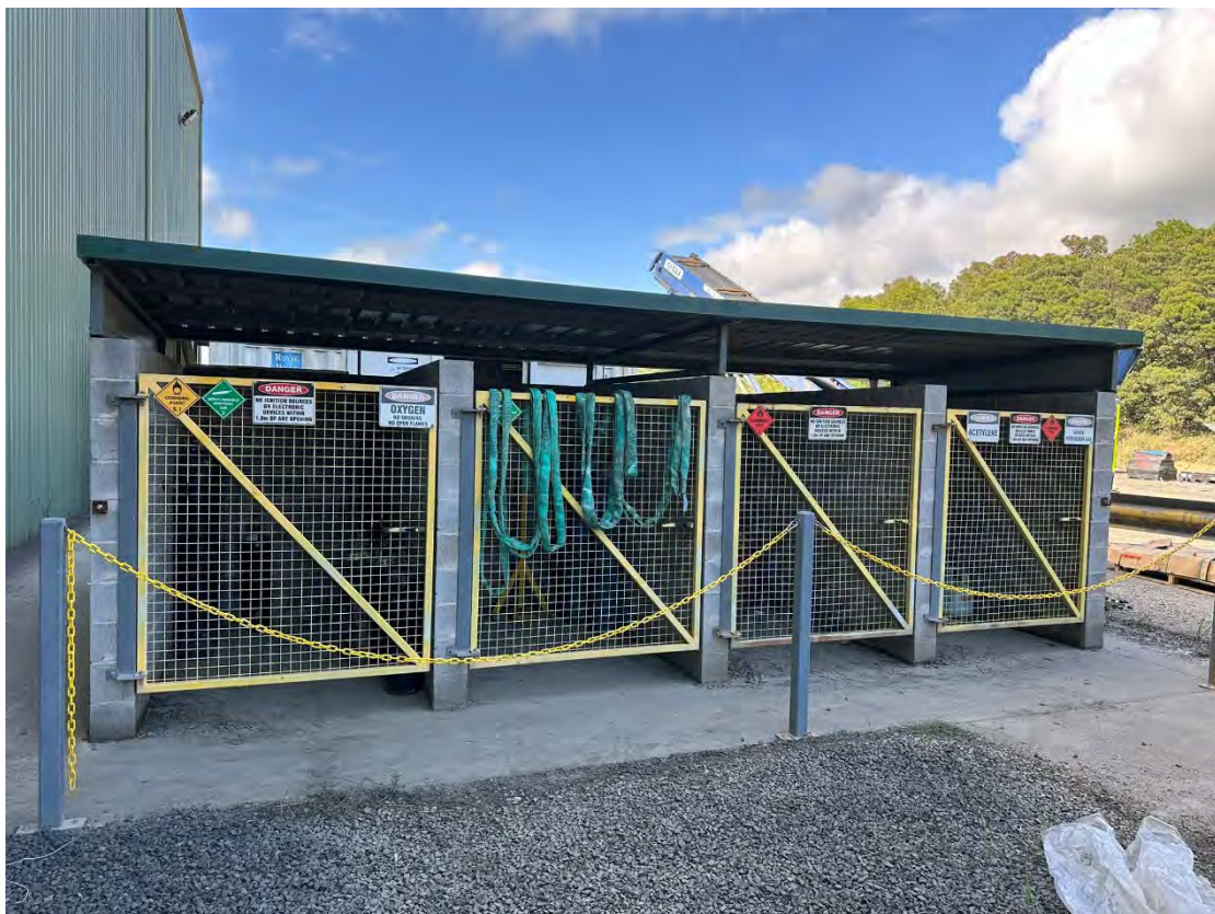
Example of dangerous good storage
