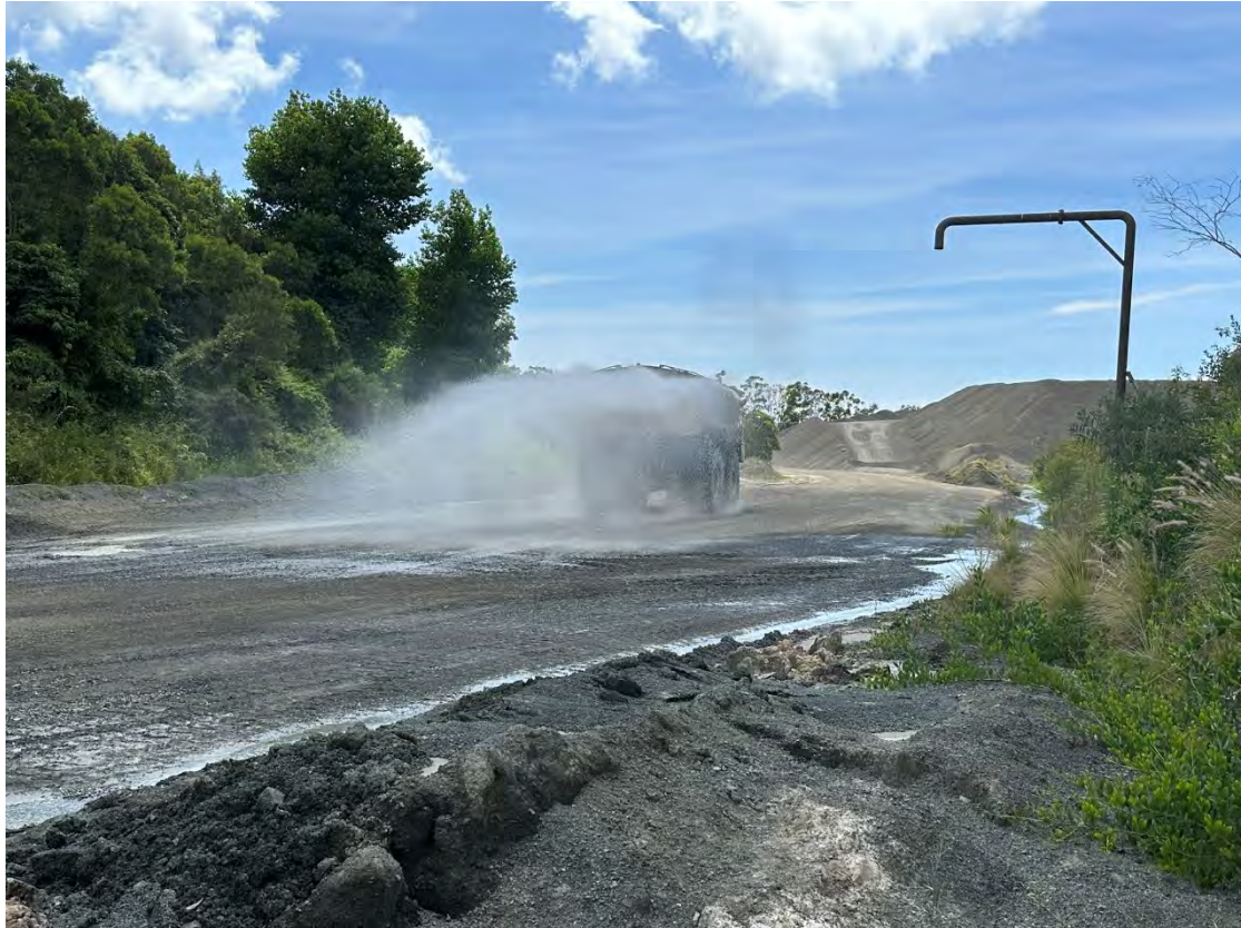
Drainage channel along internal access track into Lower Dam primary sedimentation entrance, with water cart in operation in background.
