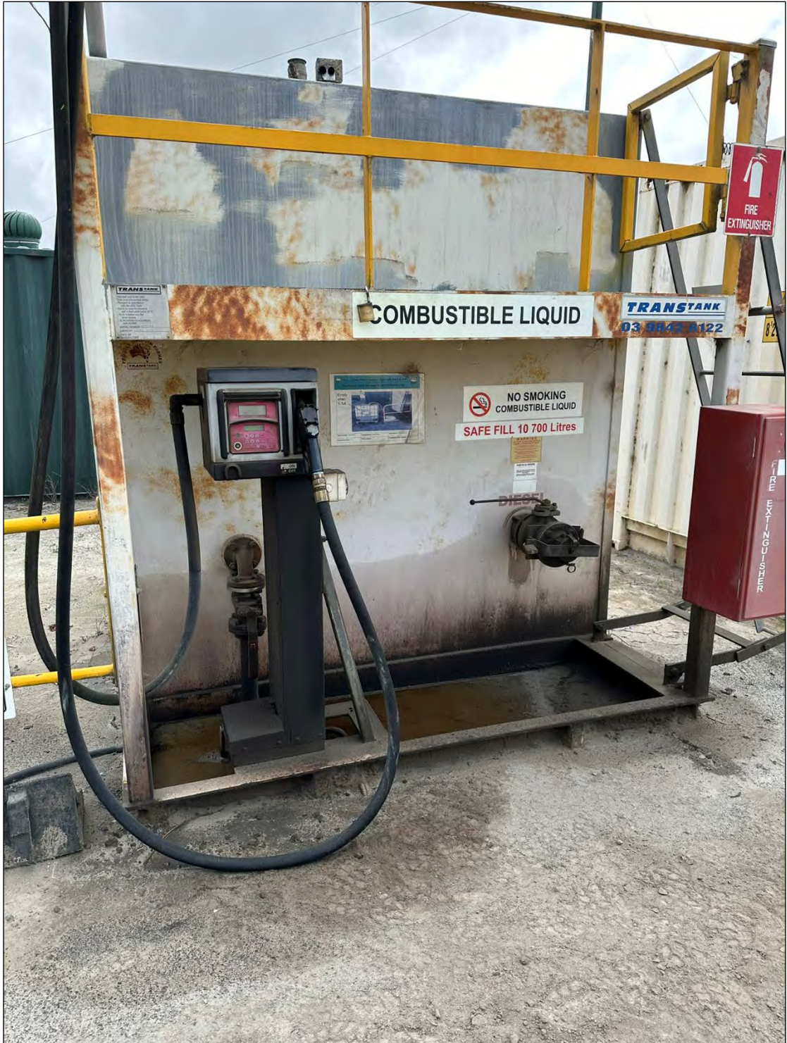
Refuelling area, bunding and fire equipment
