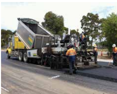
WarmPave asphalt with 15% RAP being paved on the Superway project in South Australia.
