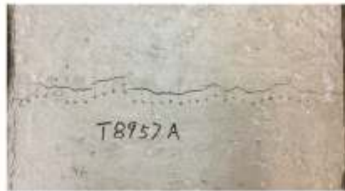
At 10mm intervals along the length of the crack
